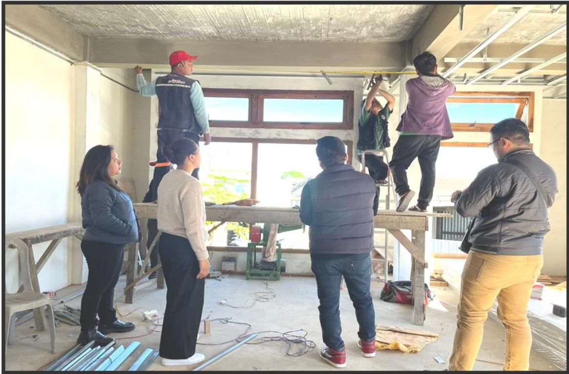
Photos: Visit of construction site during monitoring of Social Audit by Director, SAU.
